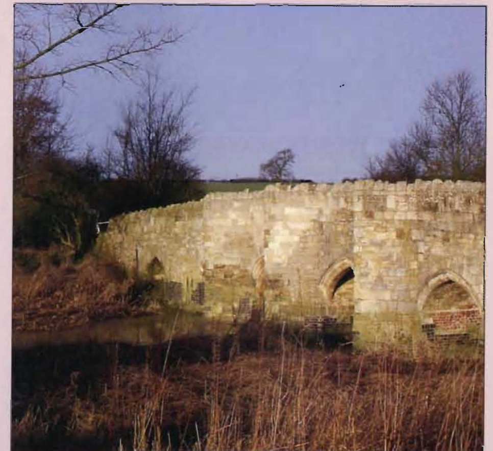
Thornborough Bridge - built in Medieval times with stone which could have come from Coombs Quarry.
